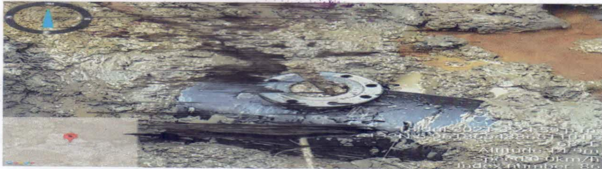
FIG. A: SHOWING 6" FLANGE INSTALLED ON THE PIPELINE BY UNKNOWN PERSON(S) FOR THEFT
